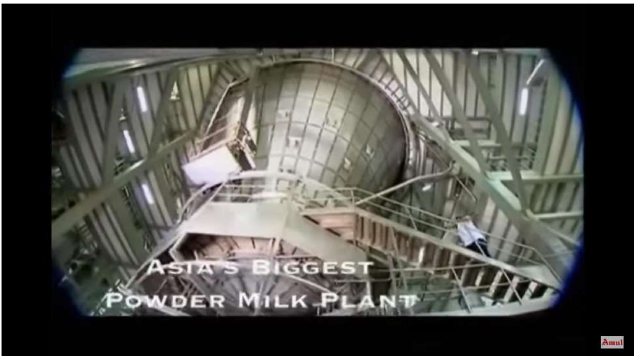
Amul Plant- Asia's Biggest Plant
