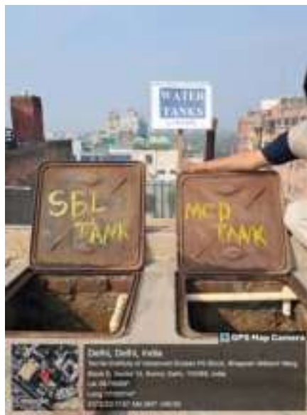
PG TERRACE WATER TANK
